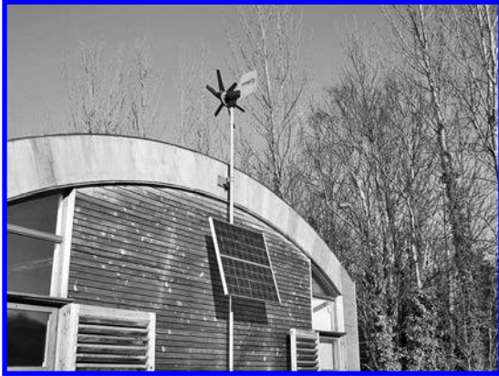
FIGURE 14. Photovoltaic solar panel on Torfaen Environmental Building.
