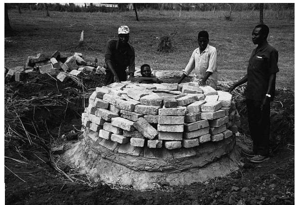
Fig. 2. Dome of a prototype underground rainwater tank in rural Uganda undergoing proof loading to 1500 kg.
